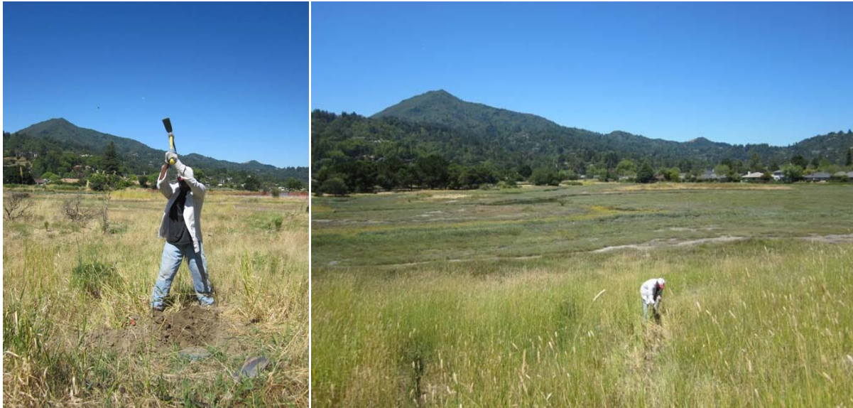
On a day where temperatures neared 100 degrees, Wayne G. digs a hole and clears Harding Grass for a new valve and drip irrigation system at Creekside Park.
