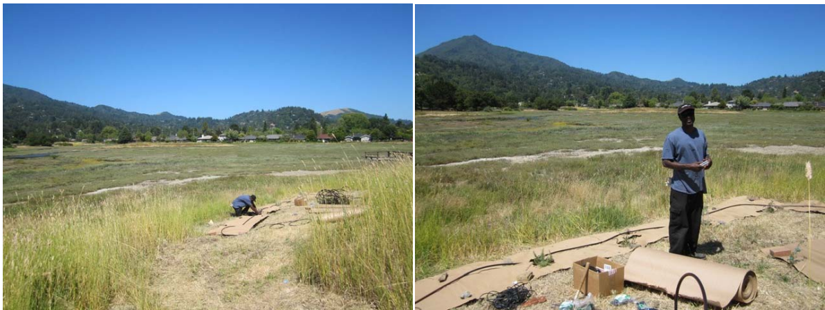
Twumasi B., aka "T", installs a drip irrigation system and cardboard to be overlaid with mulch at Creekside Park.
